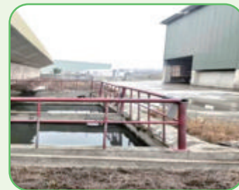
After sedimentation in the sedimentation tank, the wastewater is stored in the recovery tank and recycled for use in the factory
