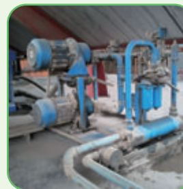
Temperature regulation of cooling water for equipment
