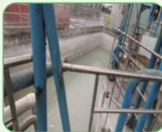
Clarification tank for tank car cleaning
